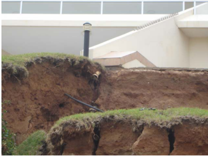
Plate 1 - Suntrap - stormwater pipe causing local erosion of bank.JPG
