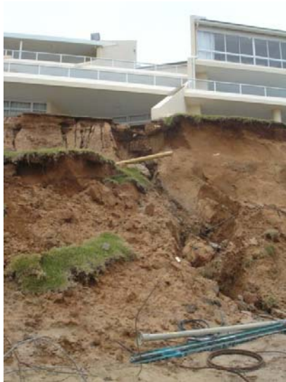
Plate 2 - Suntrap - Second stormwater pipe causing local erosion of bank.JPG
